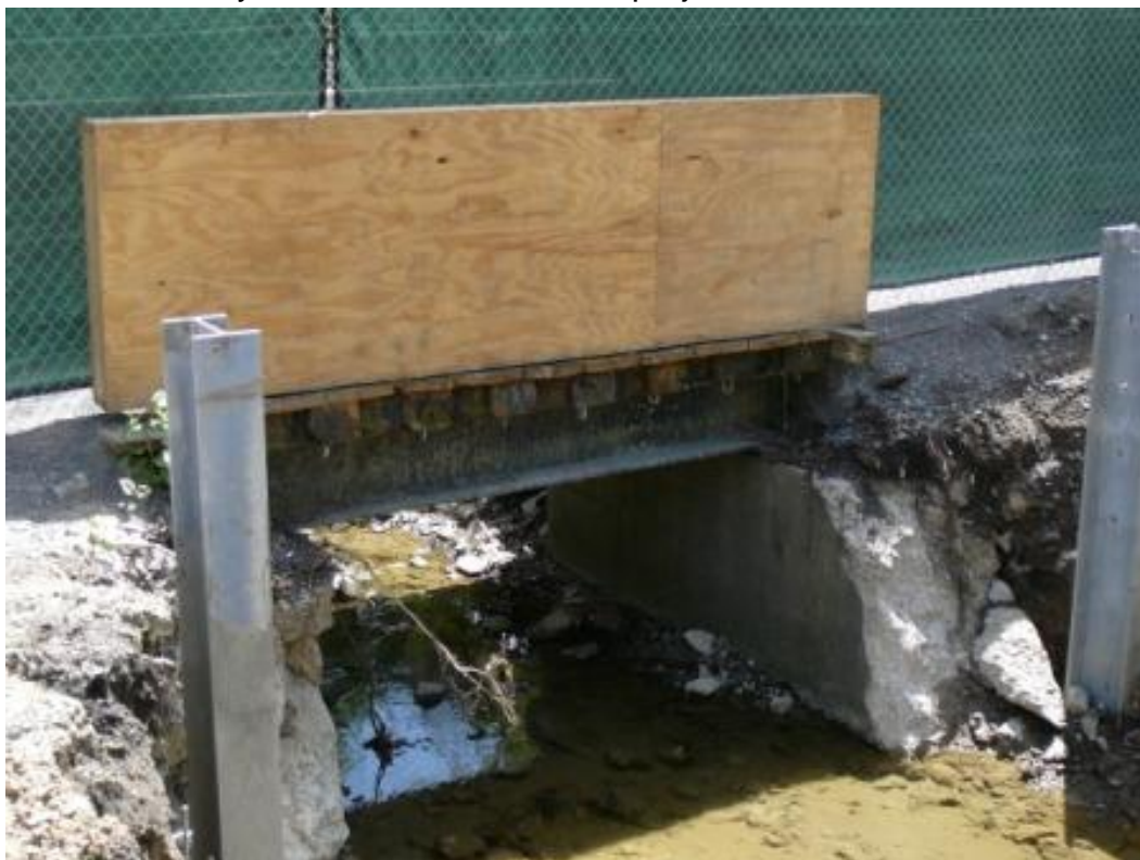
Main Line span relocated to temporary Trail on old siding RoW in May 2010. This span was removed by contractor when culvert project was finished.
