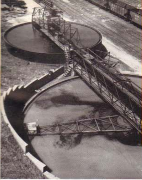
DORR THICKENER —All water from the system runs to these reservoirs. The fine coal sediment is recovered and taken back through the flotation plant.
